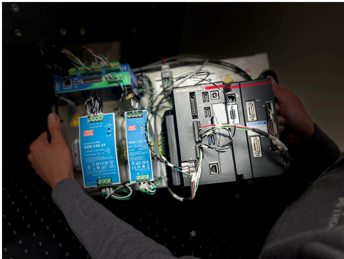
PM-1 Electrical Panel with LJ-X8002 Installed
